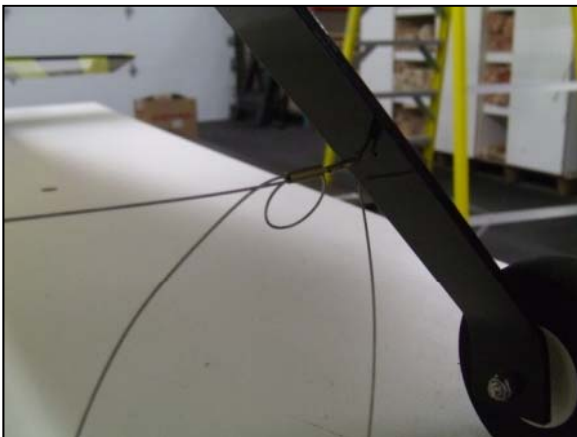
54-) Using one Brass sleeve, pass the steel cable in a “loop style” in order to make a knot into it.
